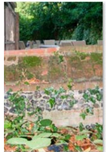
Churchyard wall poor repairs 3
